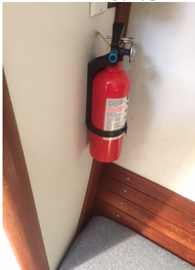
ABC: I Extinguishers- Aft cabin/
