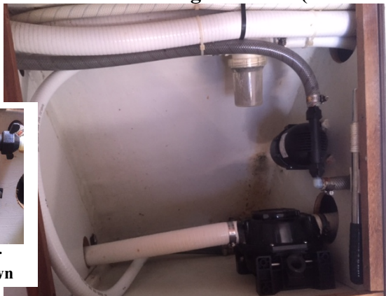
Manual holding tank pump-out w/handle
